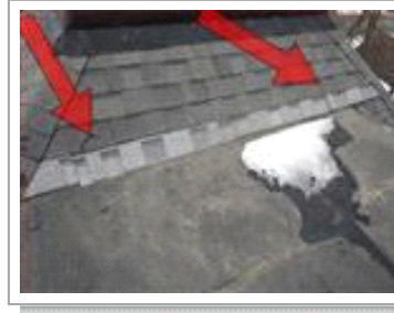
Evidence of newer repairs were found on rear of roof via newer shingles. Moreover some of the rubber membrane was loose at corners needing to be re-secured with adhesive.
