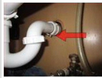
PLUMBING- Kitchen sink faucet has a slow drip/broken sprayer and the drain inside the base cabinet has a leak at a compression fitting when in use, repairs are needed.
