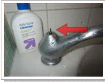
BATHROOM- Handle for the shower lever was broken/damaged, shower can be operated using a pliers to lift valve.
