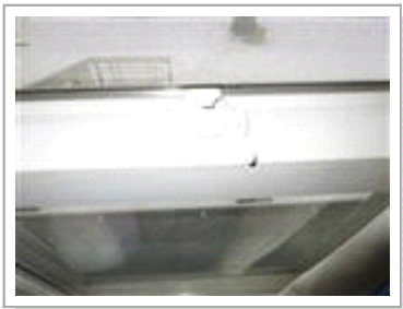
Rear window did not clasp shut when operated.
