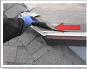
Evidence of newer repairs were found on rear of roof via newer shingles. Moreover some of the rubber membrane was loose at corners needing to be re-secured with adhesive.
