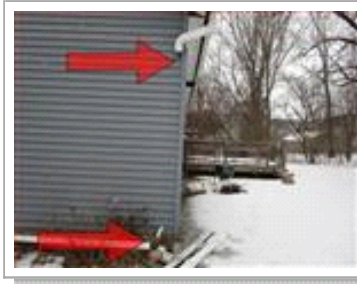
GUTTER- Down spout located on the SE corner of home was off/disconnected and laying in the snow.
