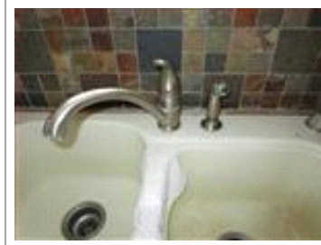
PLUMBING- Kitchen sink faucet has a slow drip/broken sprayer and the drain inside the base cabinet has a leak at a compression fitting when in use, repairs are needed.
